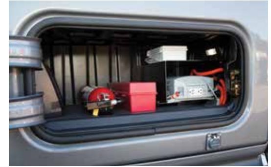
Factory-installed 1,500-watt inverter
